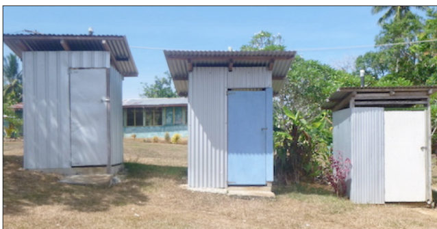
Exterior of VIP toilets. VIP toilets built by students at Lemikot Nursing School, New Ireland Province (photo by Penny Dutton)
