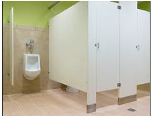
All toilet sizes. Child sized toilets and urinals are especially relevant for facilities with many child patients or visitors and for paediatric wards (photo by Facilities Net)
