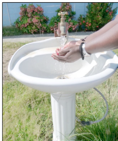
Handwashing facilities installed during COVID but lack soap
