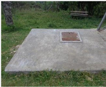
New septic tanks
