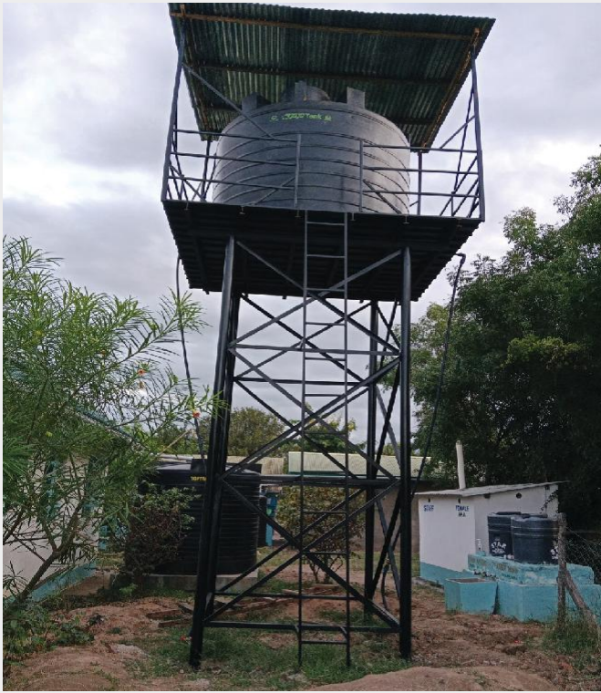
New water tank reservoir
