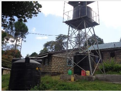
New rainwater Tanks
