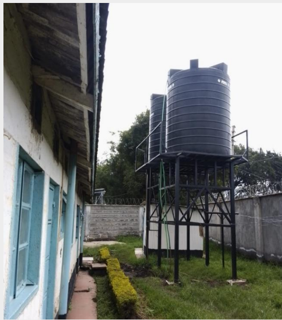
New storage water tanks
